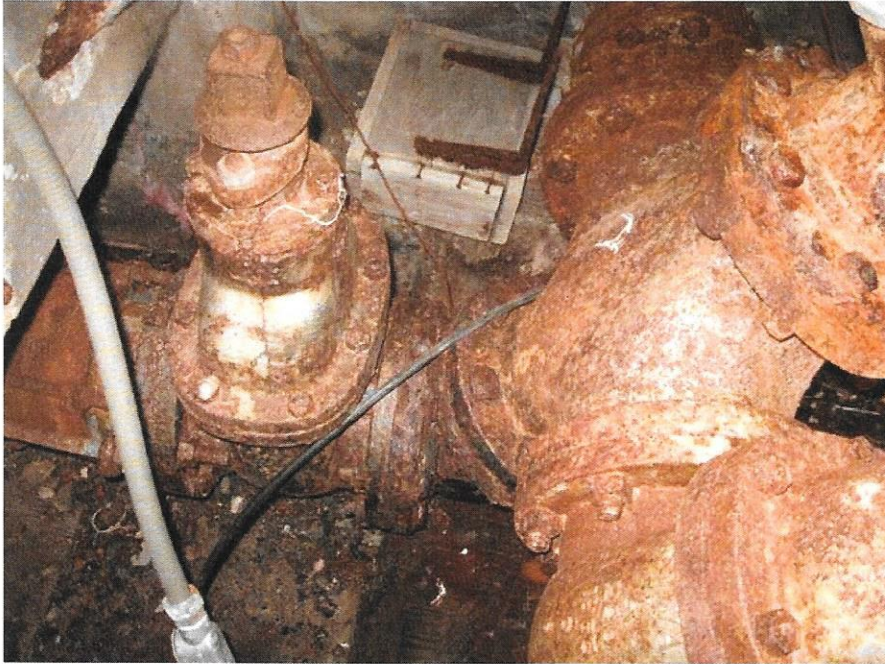
Figure 6. Piping Inside Pumphouse.
