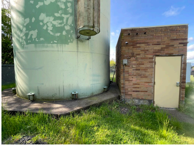
Photo 2: Well House and Reservoir
