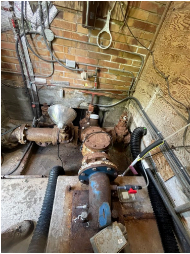
Photo 3: Well House Piping
