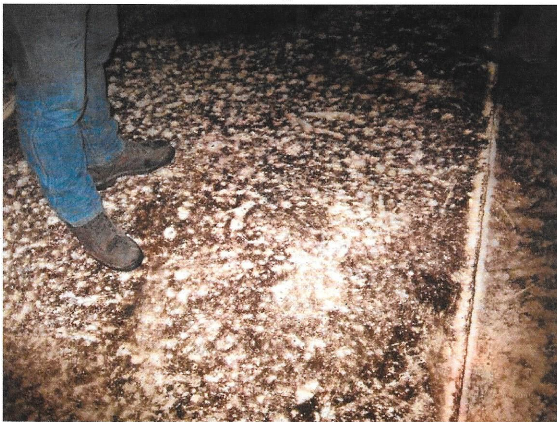
Figure 1. Reservoir Floor After Pressure Washing
