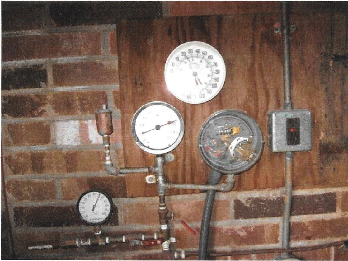
Figure 10. Interior Gauges Inside Pumphouse.
