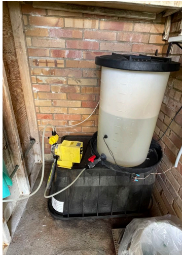
Photo 4: Well House Chlorine Room
