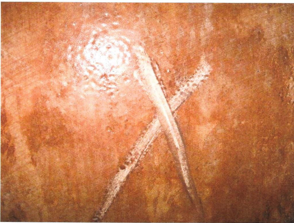
Figure 3. Interior Walls After Pressure Washing.
