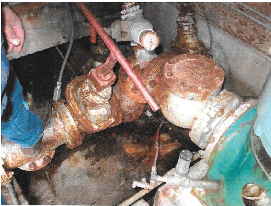
Figure 7. Piping Inside Pumphouse.
